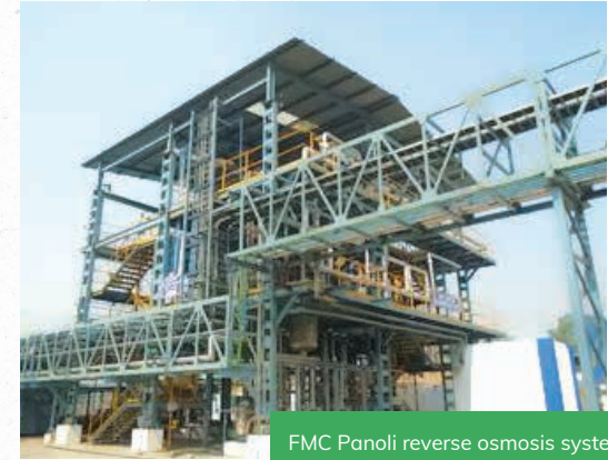
FMC Panoli reverse osmosis system
